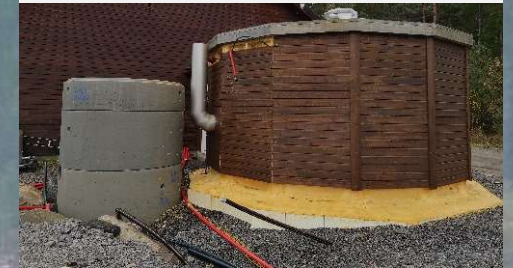
Biogas plant for cow manure since 2011, now converting to thermophilic process
