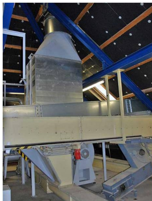
Conditioner at BAG oil mill.
