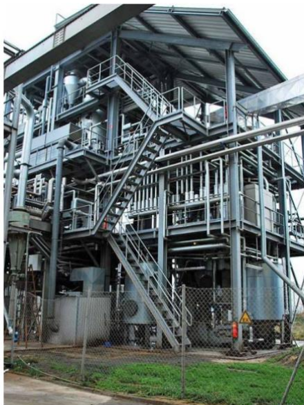
Extraction plant, BAG oil mill operations gmbH, Austria.
