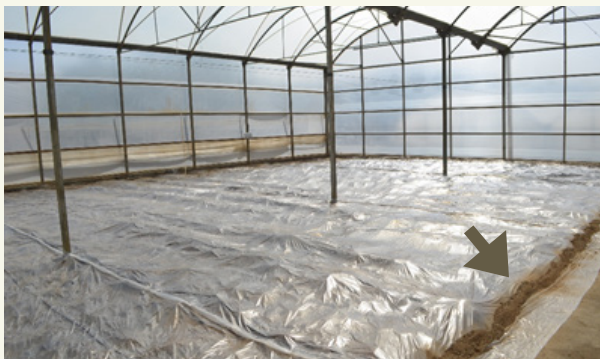
Fig. 3: After deploying the film, edges are covered with soil or other material, to avoid losses of heated air.
